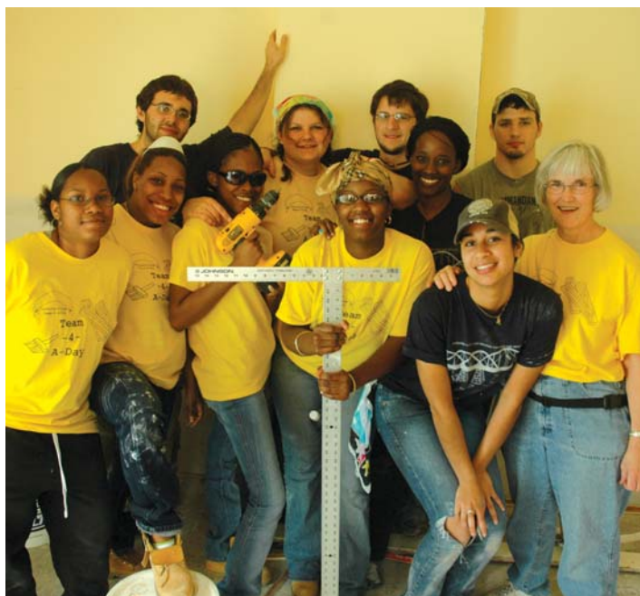
A team from La Roche works to dry wall a building on the campus of St. Augustine's, a Catholic school in New Orleans.
