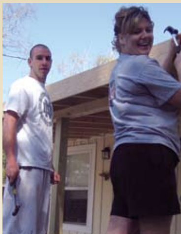
Student Chris DeCrane and Assistant Director of College Activities Katie Motycki build a roof on a porch in Mississippi.
